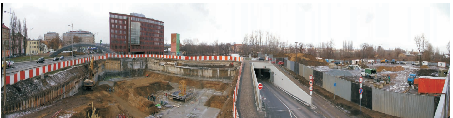
Linking garage, all four buildings is done at the level of underground parking
